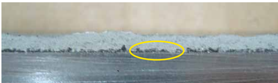
Lack of fusion is evident when the sharp edge of the vertical component can still be seen under the weld metal.
